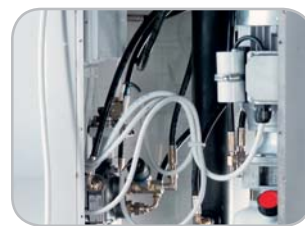
Particolare centralina e comandi Electric station and controls
